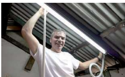
R&S employee Henrik Rausch was not the only one working up a sweat. Temperatures of up to 60 °C under the roof gables called for stamina.
