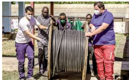
Locals and helpers from Germany work hand in hand to unwind massive cable drums. Sometimes their hands were also useful in overcoming language barriers.
